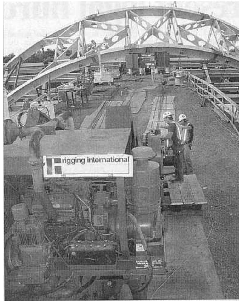
Photo/BRENT BLANCHARD, Rigging International Workers with Rigging International, based in Alameda, Calif., begin operations Friday on the south abutment of the light-rail bridge over Rancocas Creek between Delanco and Riverside.
